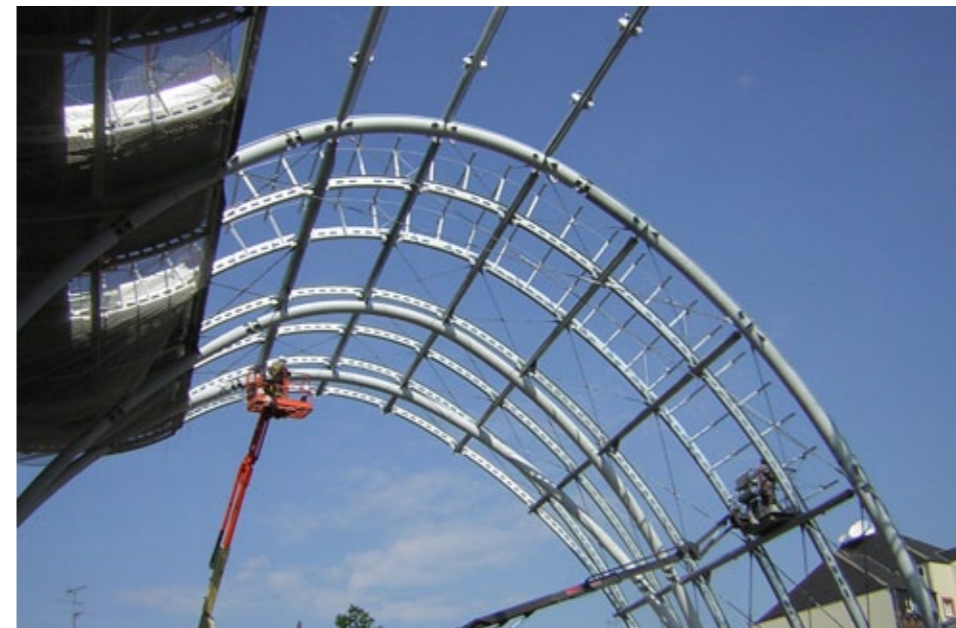
< TGV station, Orleans - FRANCE
